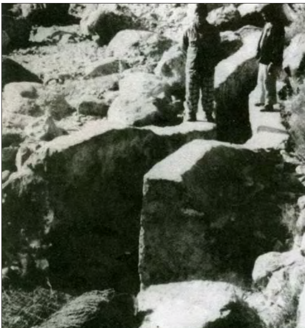
Photo 3.2 Side intake of the Galkot micro-hydro scheme, Baglung, Nepal (see Appendix C for drawing)
