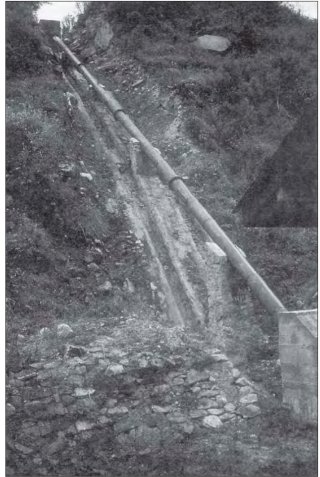
Photo 7.1 A straight penstock with four supports and an anchor block before the power house
