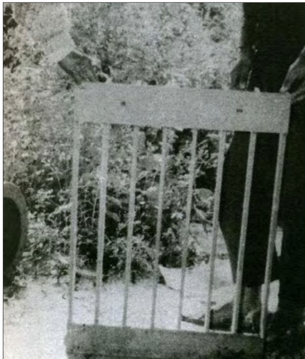
Photo 3.4 Coarse trashrack for 50 kw Galkot MHP, Baglung, Nepal. 65 mm * 10 mm flats at 75 mm centre. ( See Appendix C for the drawing )
