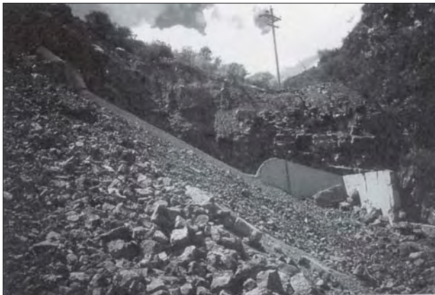
Photo 9.1 Unstable slopes are a threat to schemes. This powerhouse was destroyed by a landslide
