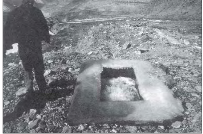
Photo 4.16 Break-pressure tank, with ice around the walls (Jhong)
