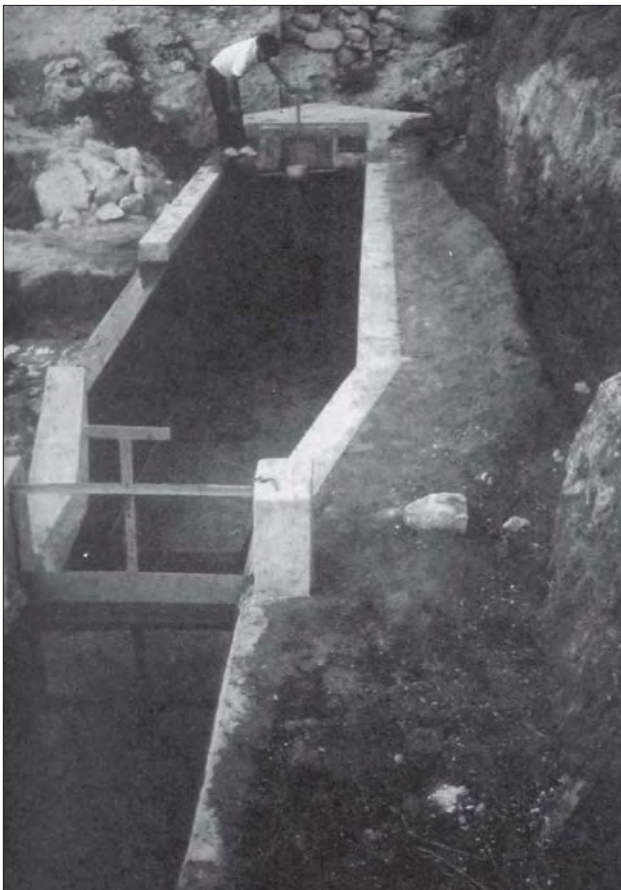
Photo 5.2 Sliding gate at settling basin entrance, Peru
