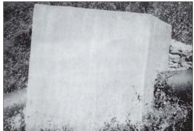
Photo 7.2 Jhankre mini-hydro anchor block for an upward vertical bend
