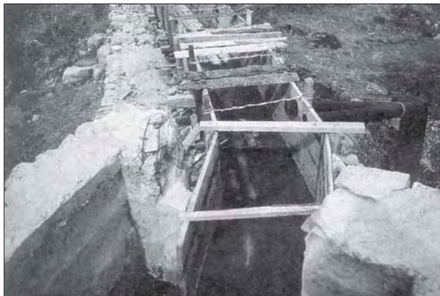
Photo 4.13 HDPE pipes provide an overflow from a timber channel (Mhapung)
