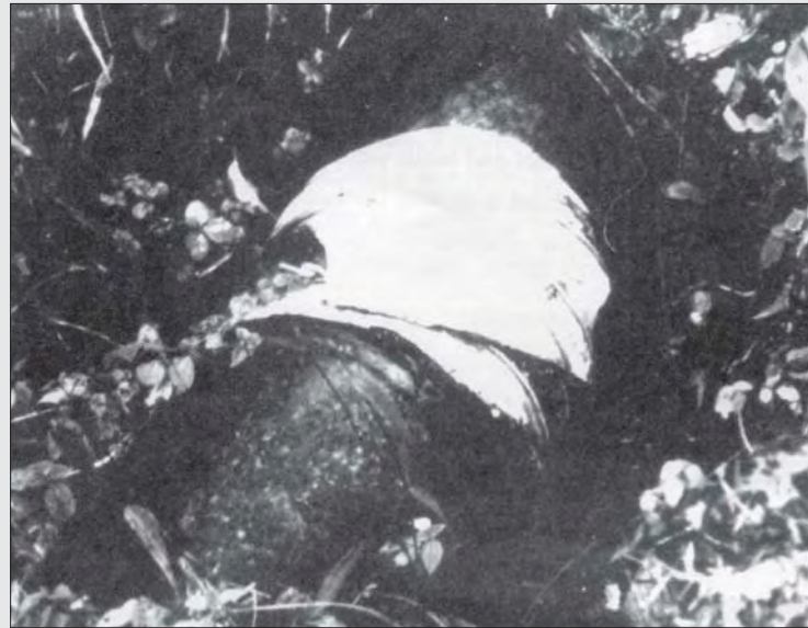
Photo 4.19 Bend prepared by cutting and welding the HDPE headrace pipe at Ghandruk
