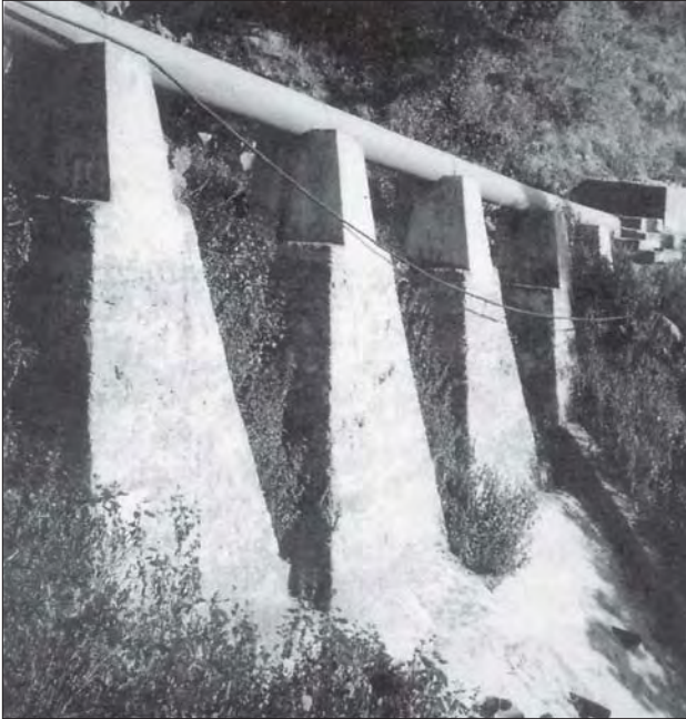
Photo 4.14 Jhankre mini-hydro penstock crossing, Dolakha, Nepal.
