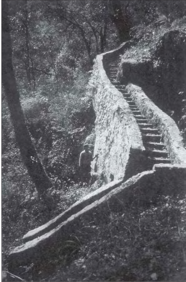
Photo 9.2 Masonry steps for energy dissipation and control of spillway water. Although costly, elaborate control is essential where slopes are vulnerable to erosion (Siklis)
