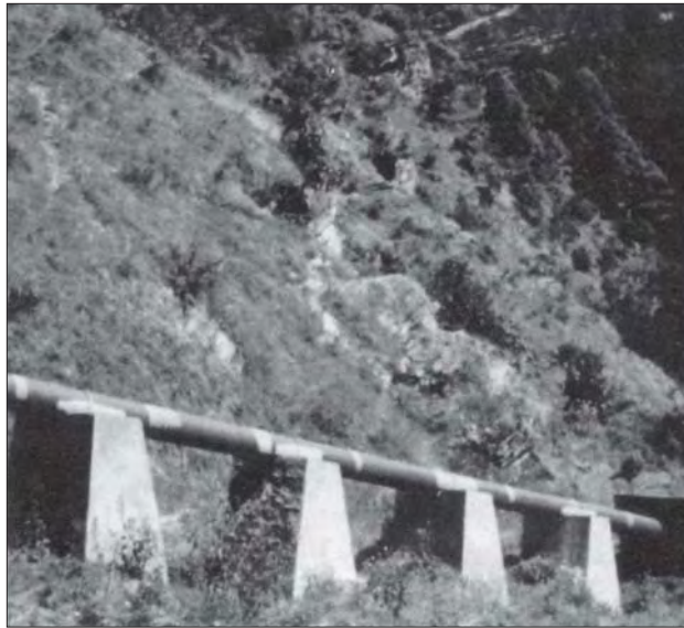
Photo 6.5 Penstock alignment high above the ground to allow access for people and cattle, Jhankre mini-hydro
