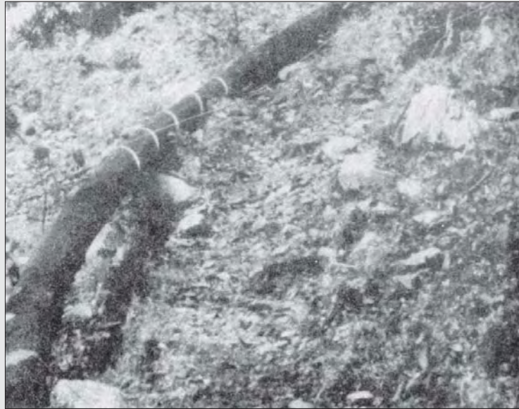
Photo 4.18 HDPE headrace pipe along unstable alignment, Ghandruk micro-hydro scheme, Nepal.
