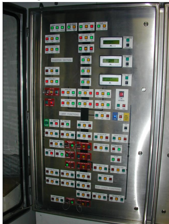
Figures 4.8.2 and 4.8.3. BOP control panels on the rig floor and bridge.
