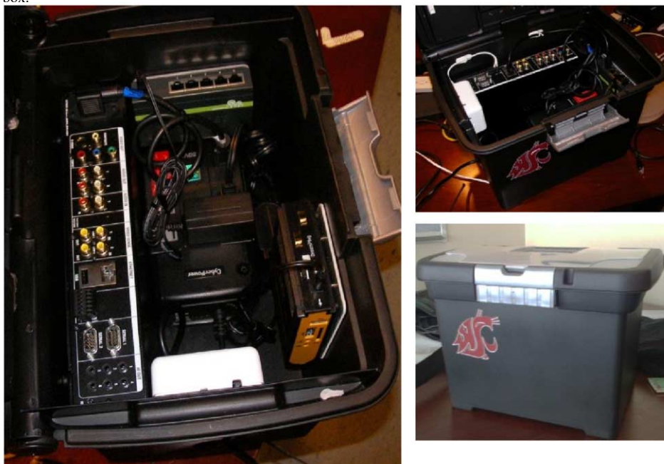
Figure 3.2. CASAS smart home components for power, networking, computation and middleware stored in a box.
