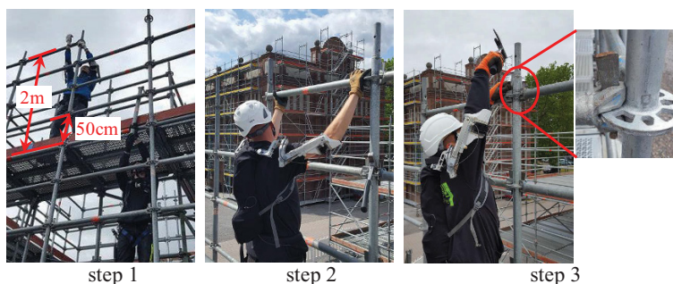
Figure 1. Installation steps of a crossbar at the highest installation level which is 2 meters high from the running board.
